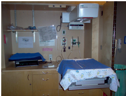
An example of temperature control from hospital
