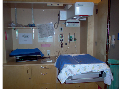
An example of temperature control from hospital
